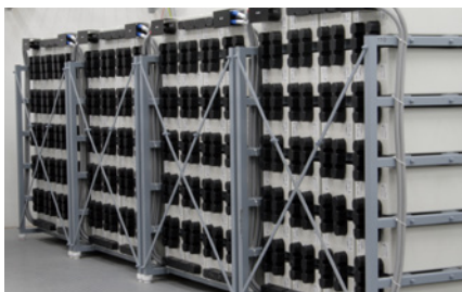
Energy Storage System
